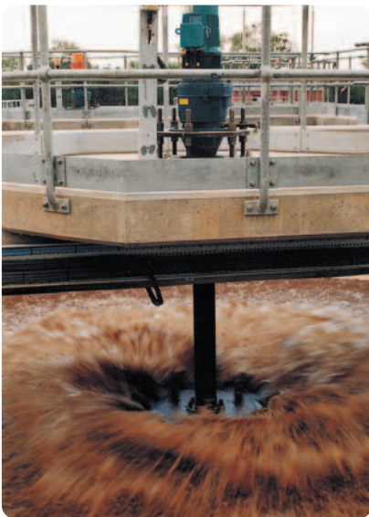
Shepshed Treatment works, Severn Trent
