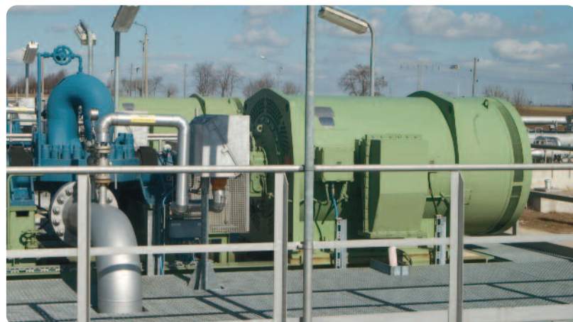
Pump drives in a pipeline booster station Powered by a Schorch, Ex de IIB T4, 1450kW, 6kV, 2 pole motor
