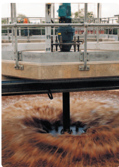
Shepshed Treatment works, Severn Trent
